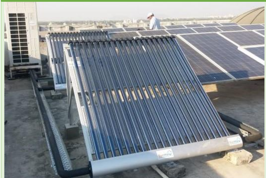
VRV system with Solar heating or Solar thermal cooling system
