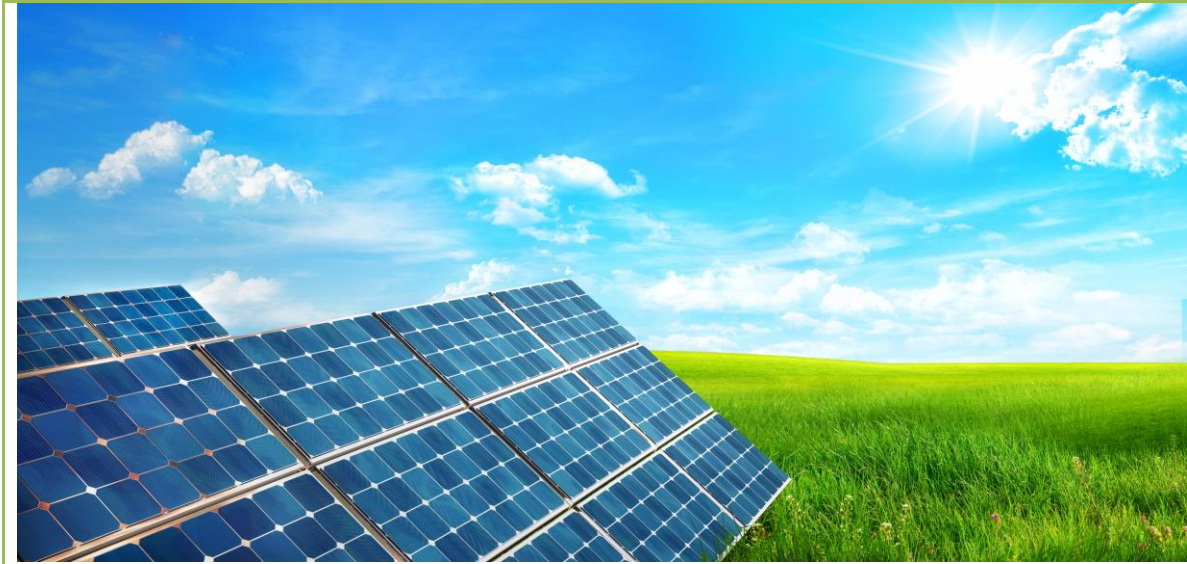
Solar photovoltaic system- with Net meter
